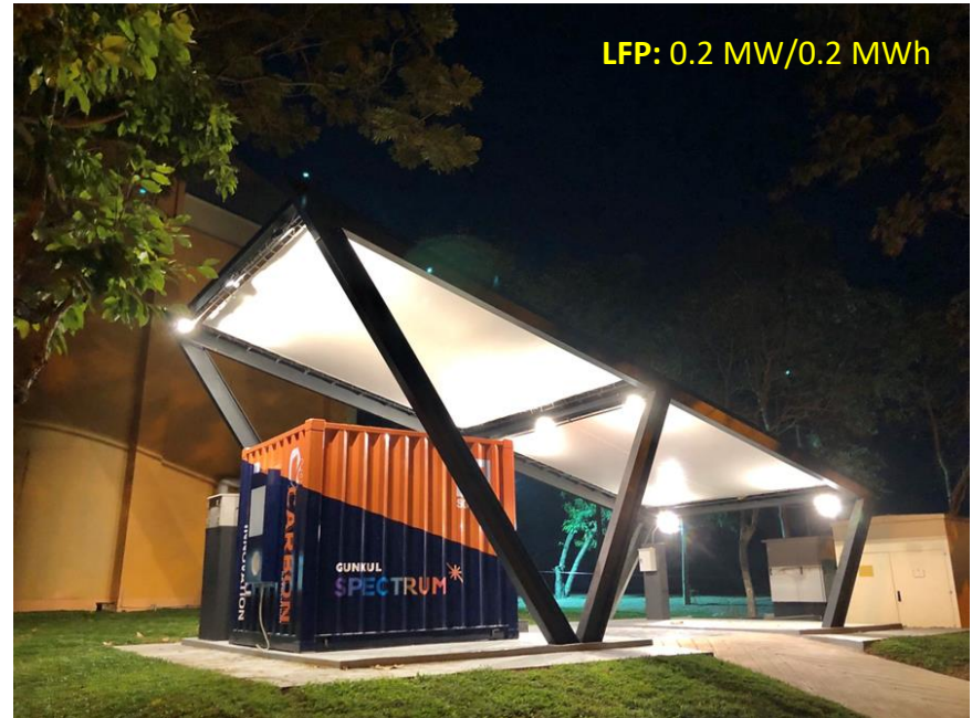
Reference: SGtech microgrid ZNE
